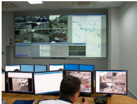
Figure 1.1: Traffic control room example.
